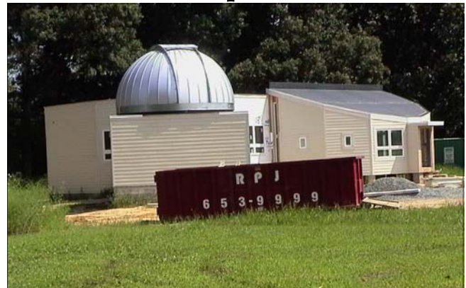
The DASEF Observatory and Environmental Outpost currently under construction at Big Oak Park near Smyrna.
